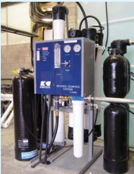
Kinetico RO System at Speirs
