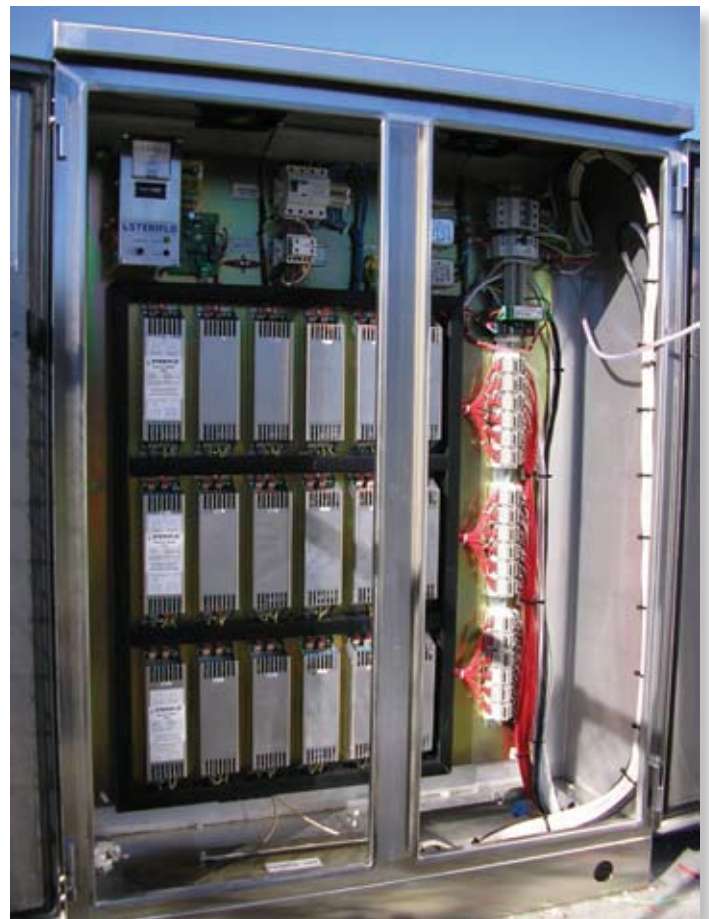
Electronic ballasts at WWTP
