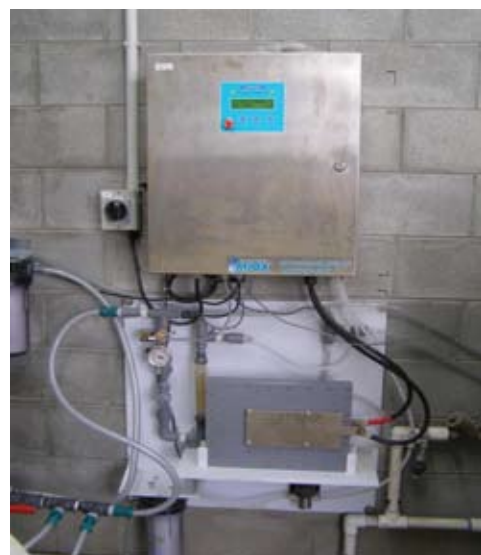
MIOX hypochlorite generator
