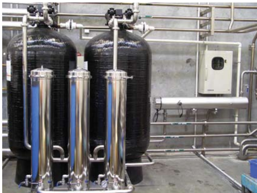
Water treatment system Christchurch juice plant
